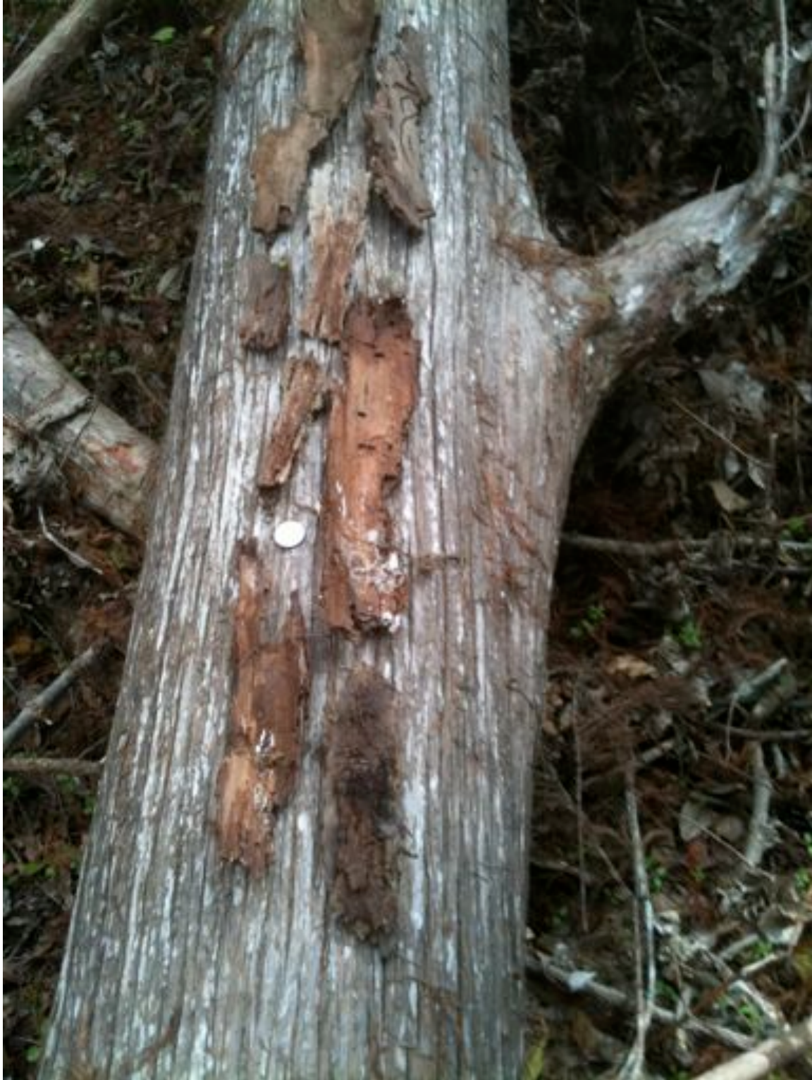
Figure 18. Bark chips found under scaled snag, Three Rivers WMA. Reference object is a quarter, diameter of just under 1”.
